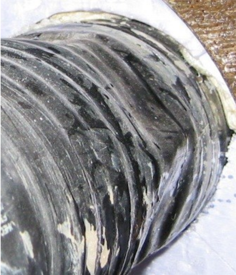
Figure 86, Jacket deformation due to incorrect selection of the annular seal
