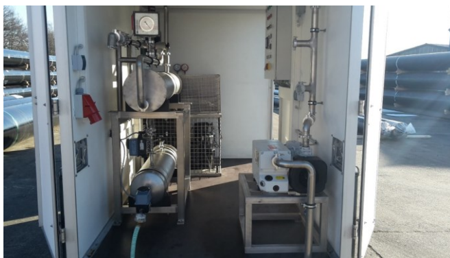
Figure: Mobile vacuum pump stand
